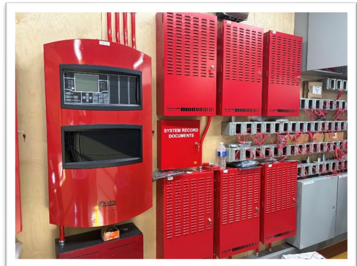
Installed Fire Suppression Equipment at Forrest Frick Pumping Plant
