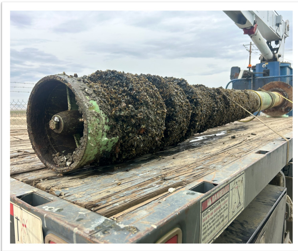
Dead Mussels on From Treatment Vertical Pump at N55-P1 Unit #7
