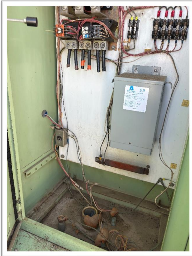
Motor Control Housing Vandalism at Tejon Well #88
